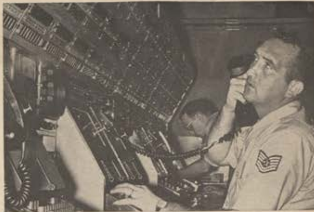
Technician in AFCS channel and technical control facility on island of Guam checks circuit status indicator boards to ensure that lines are open for users of Defense Communications System between the US and bases in Far East.
