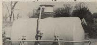
1,300 Gallon Hydrogen Peroxide Storage Tank
