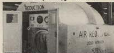
500 Gallon Liquid Oxygen Storage Tank
