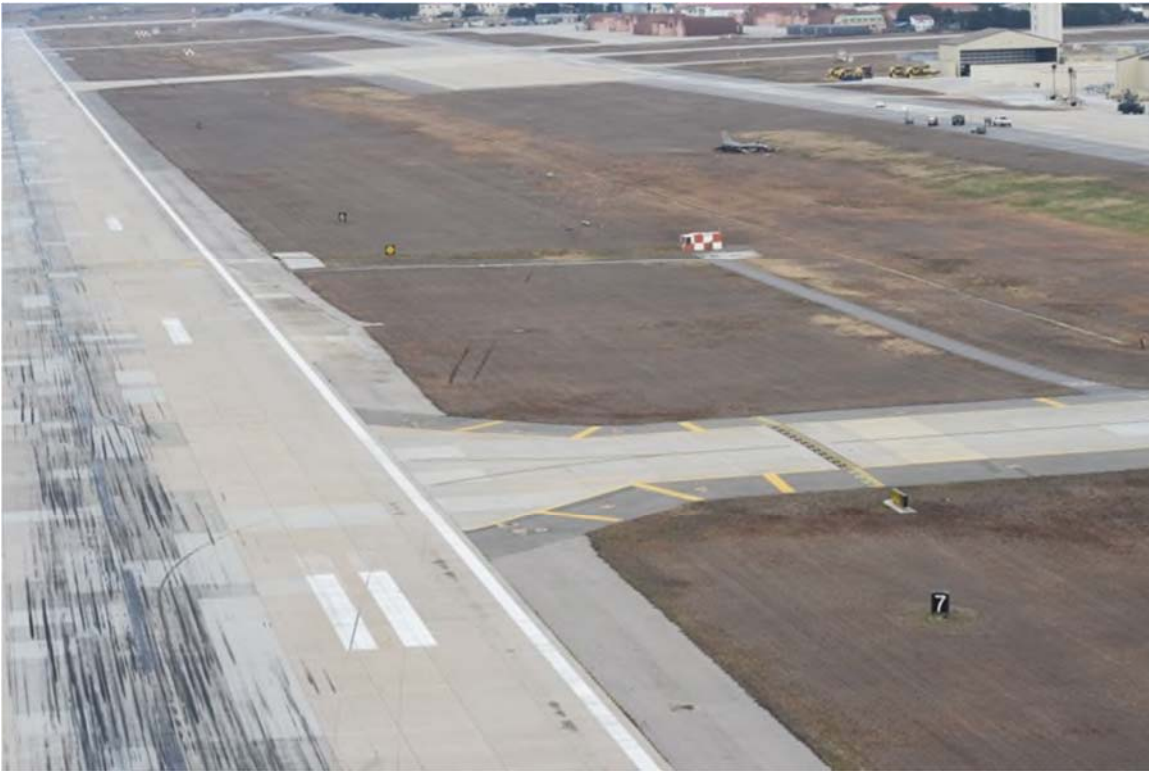
Image 10. Mishap Site Looking North; Runway Witness Marks Leading Into the Grass (Tab Z-7)
