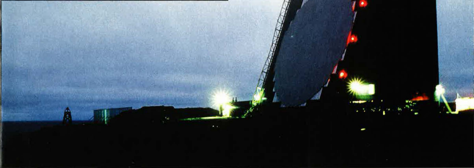
The Cobra Dane radar at Eareckson Air Station on Shemya Island, Alaska. It can detect objects 2,000 miles away and provides data for the Space Surveillance Network and the Ballistic Missile Defense System.
