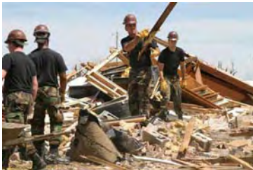
The Kansas Air National Guard works hard to remove debris from Greensburg High School after it was hit by a massive tornado May 4.
