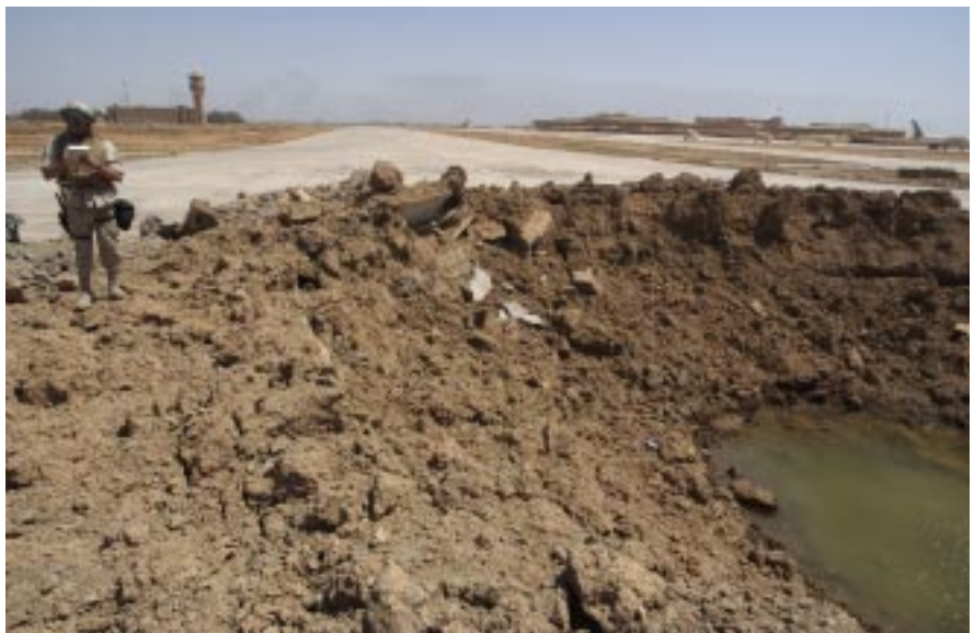
Below, engineers from the 823rd RED HORSE unit, Hurlburt Field, Fla., repair a hole in the runway.
