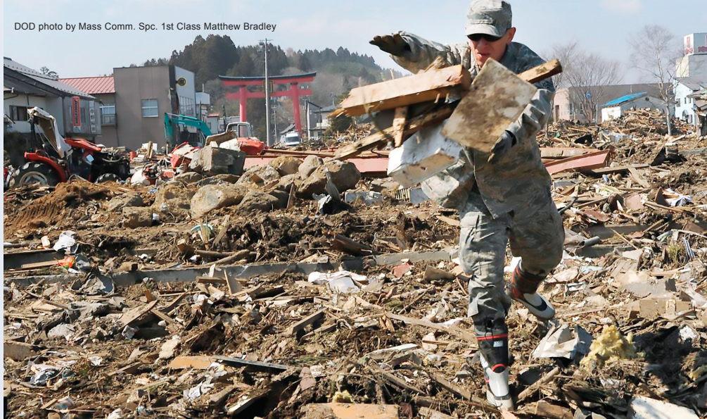
SrA. Christian Coleman cleans up debris in Noda, Japan, in 2011 during Operation Tomodachi, the humanitarian assistance-disaster relief effort undertaken after a devastating 9.0 earthquake.
