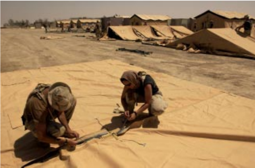
Members of an Air Force expeditionary services unit construct tents at Tallil AB, Iraq. USAF is developing a force module approach to organize the personnel needed to set up new bases for operations.
