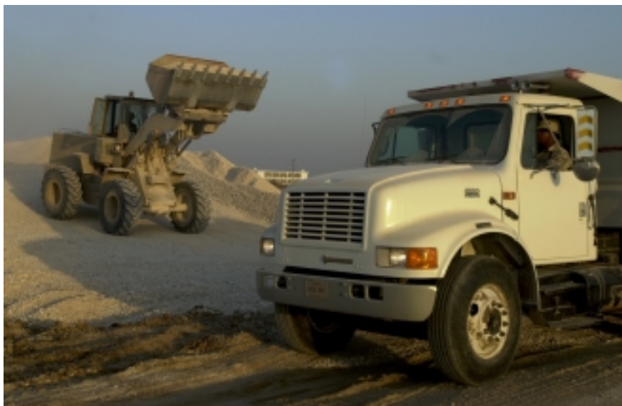
It takes some work to build a base from scratch. SSgt. LeRoy Huyghue III waits in his dump truck for TSgt. Dale Scott to deposit a load of gravel destined for a tent city the 823rd RED HORSE Squadron is creating at a forward location.
