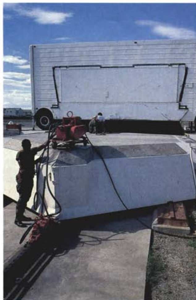
Training plays an important role in the lives of both maintainers and crews. Here, Sgt. Bill Matthews (left) and Amn. Jonathan Wood (right) train topside at Malmstrom's T-9 facility. The 110-ton blast door covering the top of the silo must be closed with a hydraulic unit known as a "pipe pusher" that moves the door three inches at a time.
