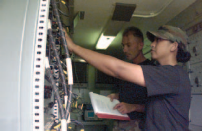
AIC Rachel J. Shields, a Satellite Communications Apprentice and SSgt Thomas A. Schell, a Satellite wideband Communications Journeyman both with the 31st Communications Squadron perform an operational check on equipment in a SATCOM van.
