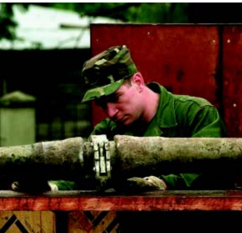
An environmental engineer with the 5th Civil Engineering Squadron, Minot AFB, ND, checks the connection of two hoses. He was part of a multiservice construction crew building a school in Teguiipa, Bolivia.
