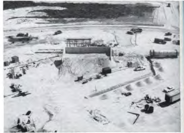
Unlike Atlas sites, each of which stores its own missile fuel, groups of three Titan I launchers are served by a central tank, while portable tankers fuel Titan IIs. Here construction begins on the still more advanced fuel storage system for the new Titan III.
