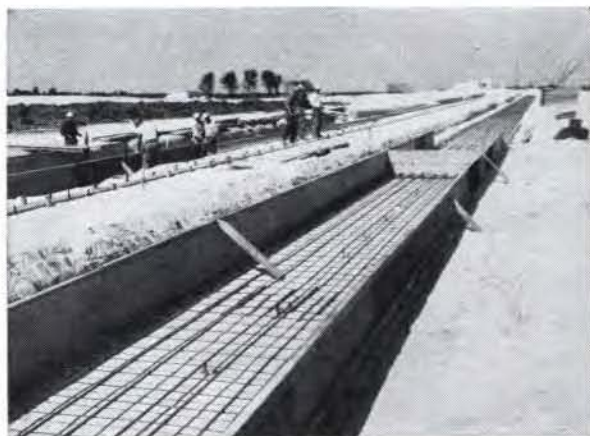
Concurrency concept in site construction is demonstrated in this view at Cape Kennedy, Fla., where workmen are preparing railbeds leading from Titan III booster assembly area to launch pad, while the components of Titan III are still under development.
